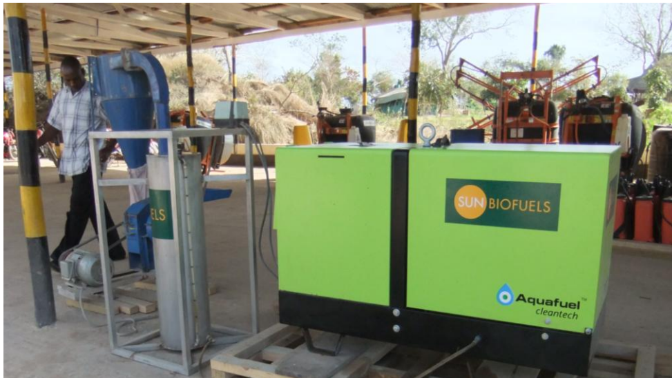
A 10kW generator modified by Aquafuel Research to run on pure Jatropha oil. The unit is being tested by SBF in Tanzania for practical applications such as powered flour mills (shown above). It has the added benefit of utilising exhaust waste heat to purify water to drinking quality
